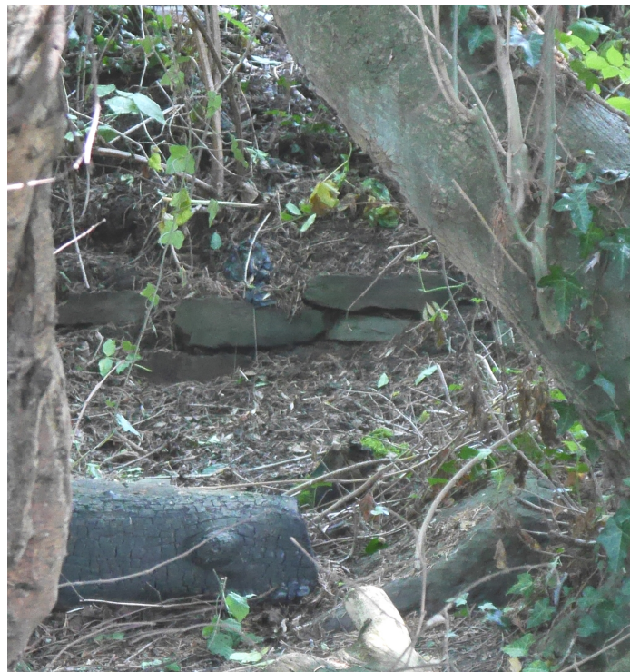
Surviving masonry in the southeast wall (with a large, squared stone in the foreground).
