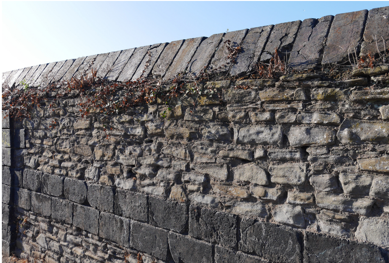
The smooth top line of the wall is illustrated here with panel 10 (photo 12 July 2025).
