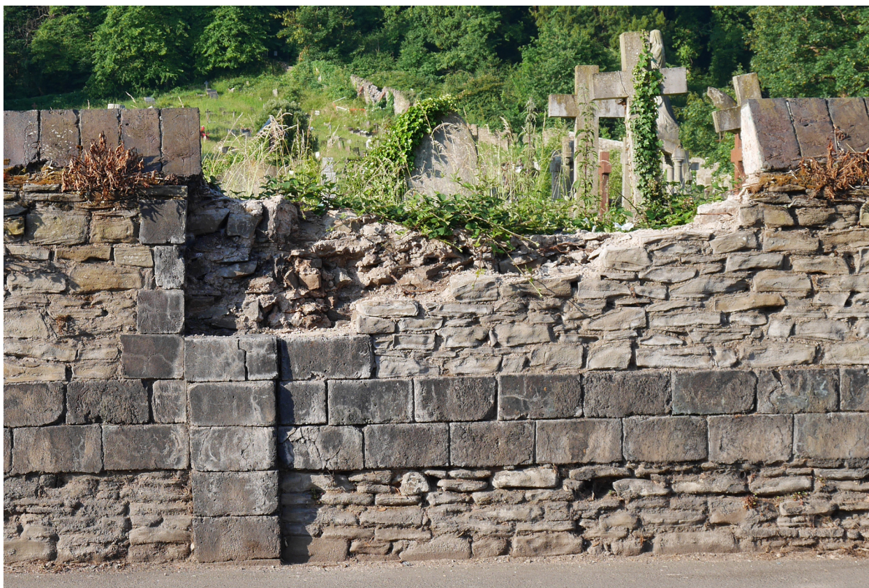
A few stones fell in January 2025, and a substantial part was then dismantled (photo 19 June 2025).
