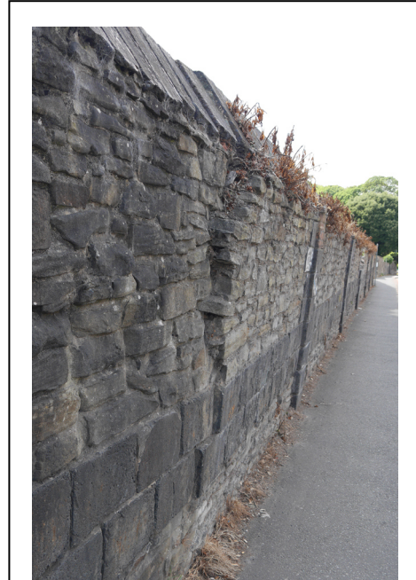
Portion of the wall to the left (east) rebuilt to make it more vertical (photo 7 July 2025).
