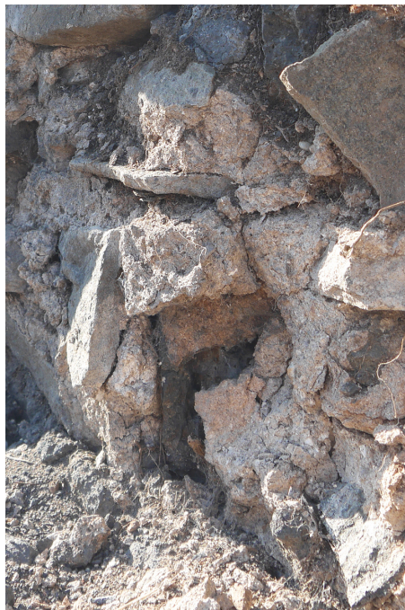
Mortar exposed by the demolition after the minor collapse in January 2025 (photo 12 July 2025).
