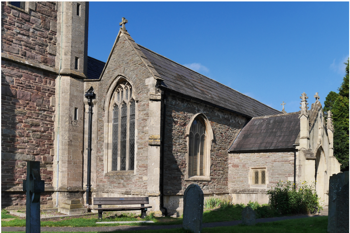
Glass fragments were found outside the two large windows at the western end of the south aisle (between the tower and south porch).
