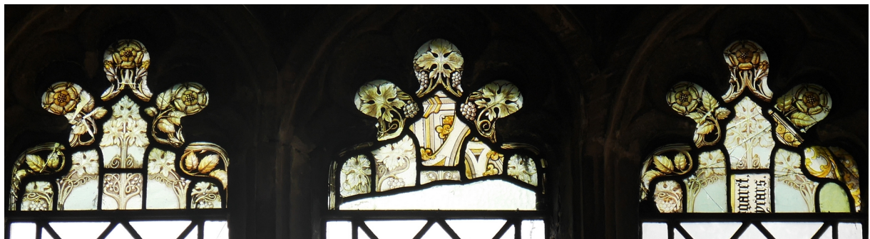
Detail of the window on the south wall between the porch and west end. These fragments of stained glass were salvaged from the window shattered by the WW2 bombing, carefully selected for suitability, and reused in this high part of the current window. The uppermost parts of the window depicting seraphim escaped blast damage, presumably because those panels had too small a surface area for the pressure wave to buckle and break them).
